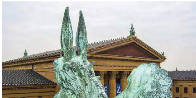
The lightning protection system is part of the Museum's comprehensive system to protect the cultural assets it houses. (The bronze acroterion in the foreground is on the roof of one of the Museum's wings.)
