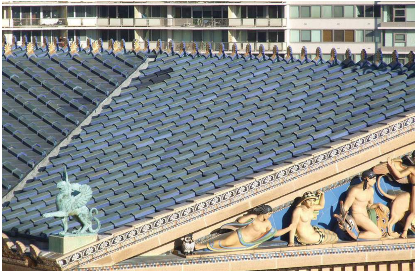
The bronze acroteria at the corner of the roof act as strike termination devices. Photo courtesy of LF Driscoll.
