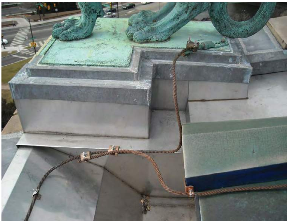
The bronze griffin protects the Museum by safely conducting lightning strikes into the ground via copper cables that are UL-listed for use in lightning protection systems. Photo courtesy of Warren Lightning Rod Co.
