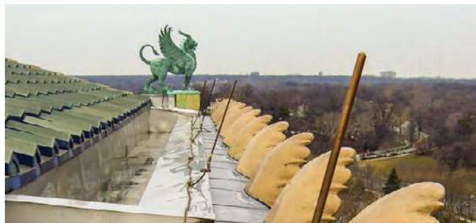
Air terminals were set on pedestals so they could reach above the decorative eave ornaments. The pedestals are set back from the roof edge and the air terminals are inclined to reach above the ornaments. Hidden behind the ornaments, the air terminals are almost invisible from below.
