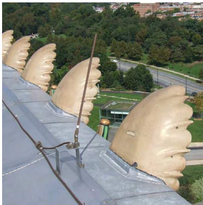
Air terminals were set on pedestals so they could reach above the decorative eave ornaments. The pedestals are set back from the roof edge and the air terminals are inclined to reach above the ornaments. Hidden behind the ornaments, the air terminals are almost invisible from below. Photo courtesy of Warren Lightning Rod Co.
