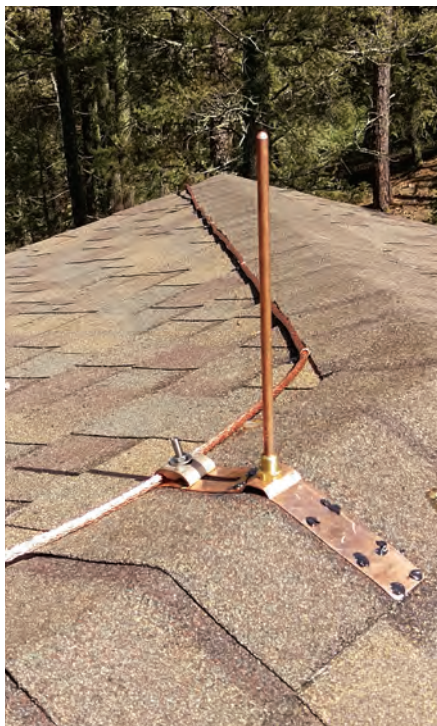
Figure 5 — Existing buildings can be retrofitted with lightning protection systems. [Photo courtesy of Mr. Lightning]
