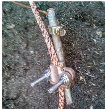
Figure 2 — The braided copper cable and large clamp are UL-listed for lightning protection and are much larger than the wire and clamp (near the top of the ½-inch-diameter grounding rod) required for ordinary household grounding. The two grounds are bonded to create a common ground point. [Photo courtesy of East Coast Lightning Equipment, Inc.]
