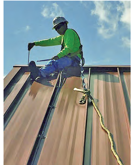
Figure 8 — Because much of a lightning protection system must be installed on rooftops or other high locations, it is advisable to have a trained professional with adequate protective gear do the work. [Photo courtesy of Labeled Lightning]
