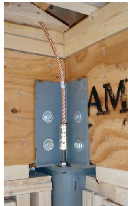
Figure 6 — A professional lightning protection installer can show you how to reduce the cost of an LPS. Here, for example, a conductor from the roof is connected to a steel column that acts as the conductor to the floor level and an external ground system. [Photo courtesy of Priestley Lightning Protection, LLC]
