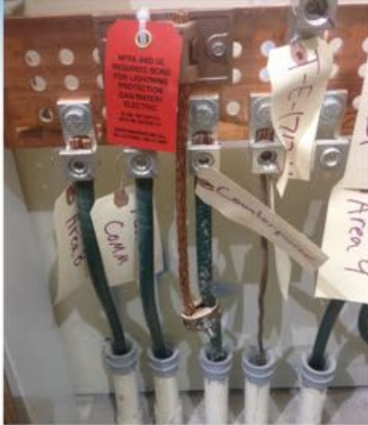
Figure 3: Lightning can exceed 3 million V and protecting structures and equipment from lightning is not covered in the electrical codes. Lightning protection system (LPS) should be designed and installed by individuals certified by the Lightning Protection Institute and using equipment specifically listed for lightning protection systems. This copper grounding bar is used to create a common ground point where the LPS and the grounds for other building services can be interconnected. Courtesy: East Coast Lightning Equipment Inc.
