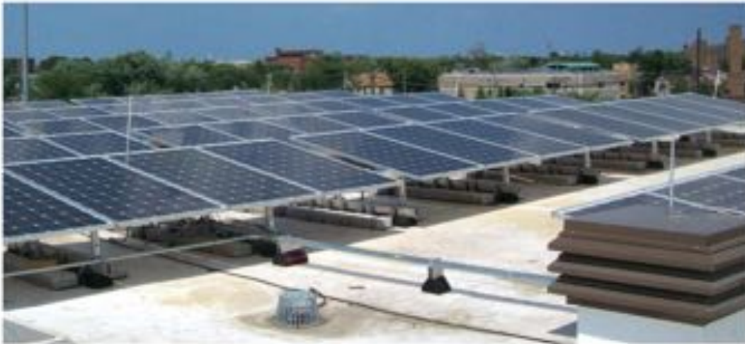
Figure 4: Photovoltaic equipment, such as this solar collector array on a municipal building, is typically installed in locations prone to lightning strikes. Courtesy: East Coast Lightning Equipment Inc.
