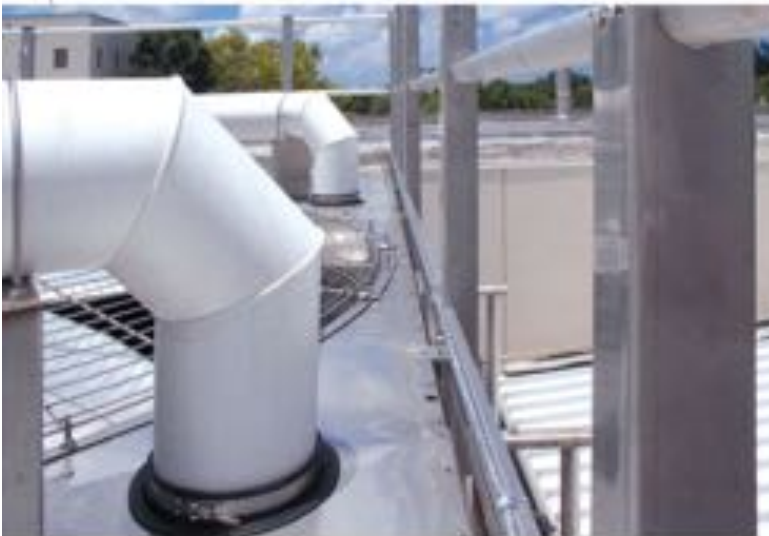
Figure 2: The physical plant director of this hospital said he can't accept the risk of lightning damage when someone could be on the operating table. The railings around this rooftop equipment acts as a strike termination device and is used in lieu of conventional air terminals (lightning rods). The cable at the base of the railing is UL-listed for lightning protection and assures electrical continuity with the rest of the lightning protection system. Courtesy: East Coast Lightning Equipment Inc.
