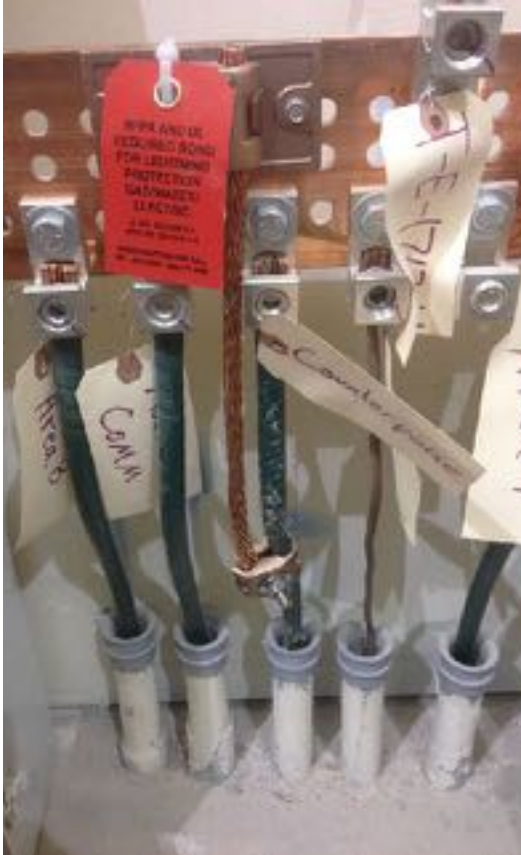
Figure 3: Lightning can exceed 3 million V and protecting structures and equipment from lightning is not covered in the electrical codes. Lightning protection system (LPS) should be designed and installed by individuals certified by the Lightning Protection Institute and using equipment specifically listed for lightning protection systems. This copper grounding bar is used to create a common ground point where the LPS and the grounds for other building services can be interconnected. Courtesy: Mr. Lightning
