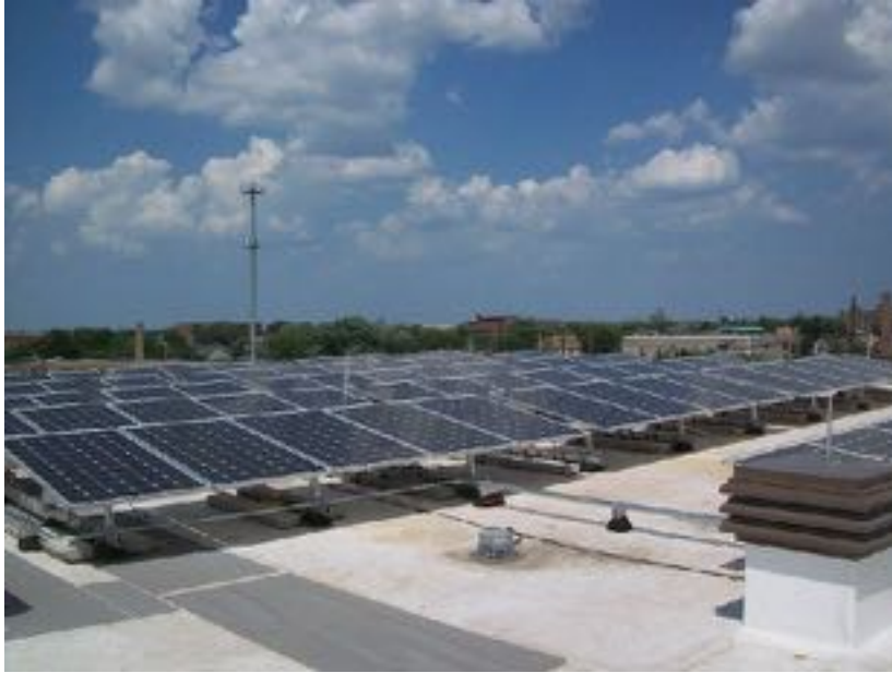
Figure 4: Photovoltaic equipment, such as this solar collector array on a municipal building, is typically installed in locations prone to lightning strikes. Courtesy: HLP Systems, Inc.
