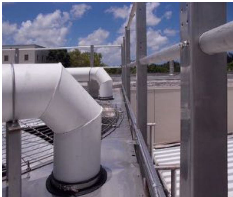
Figure 2: The physical plant director of this hospital said he can't accept the risk of lightning damage when someone could be on the operating table. The railings around this rooftop equipment acts as a strike termination device and is used in lieu of conventional air terminals (lightning rods). The cable at the base of the railing is UL-listed for lightning protection and assures electrical continuity with the rest of the lightning protection system.
