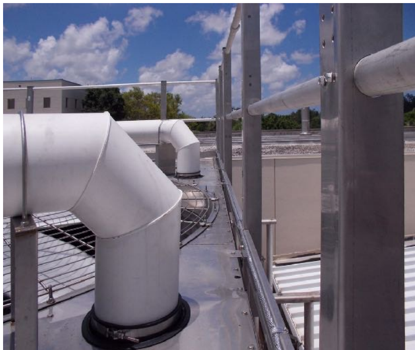
Figure 2: The physical plant director of this hospital said he can't accept the risk of lightning damage when someone could be on the operating table. The railings around this rooftop equipment acts as a strike termination device and is used in lieu of conventional air terminals (lightning rods). The cable at the base of the railing is UL-listed for lightning protection and assures electrical continuity with the rest of the lightning protection system.
