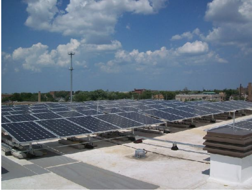
Figure 4: Photovoltaic equipment, such as this solar collector array on a municipal building, is typically installed in locations prone to lightning strikes. Courtesy: HLP Systems, Inc.
