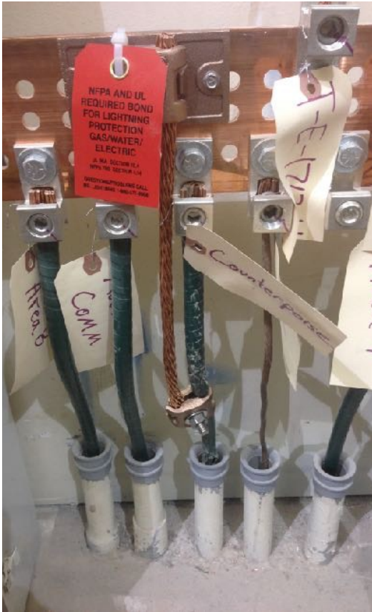
Figure 3: Lightning can exceed 3 million V and protecting structures and equipment from lightning is not covered in the electrical codes. Lightning protection system (LPS) should be designed and installed by individuals certified by the Lightning Protection Institute and using equipment specifically listed for lightning protection systems. This copper grounding bar is used to create a common ground point where the LPS and the grounds for other building services can be interconnected. Courtesy: Mr. Lightning
